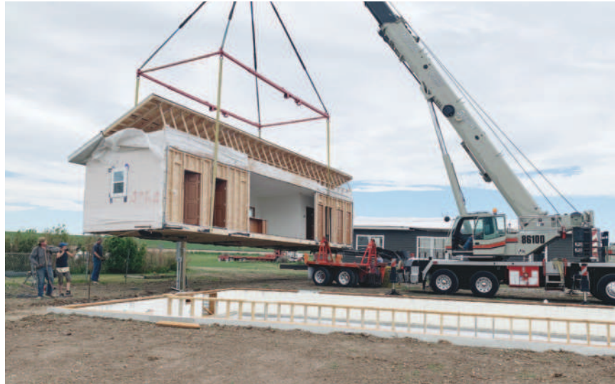
Erlandson's new modular home arrived June 17. Crews lifted the house by crane and placed it onto the foundation before completing its assembly. Photo courtesy of Carla Allen
