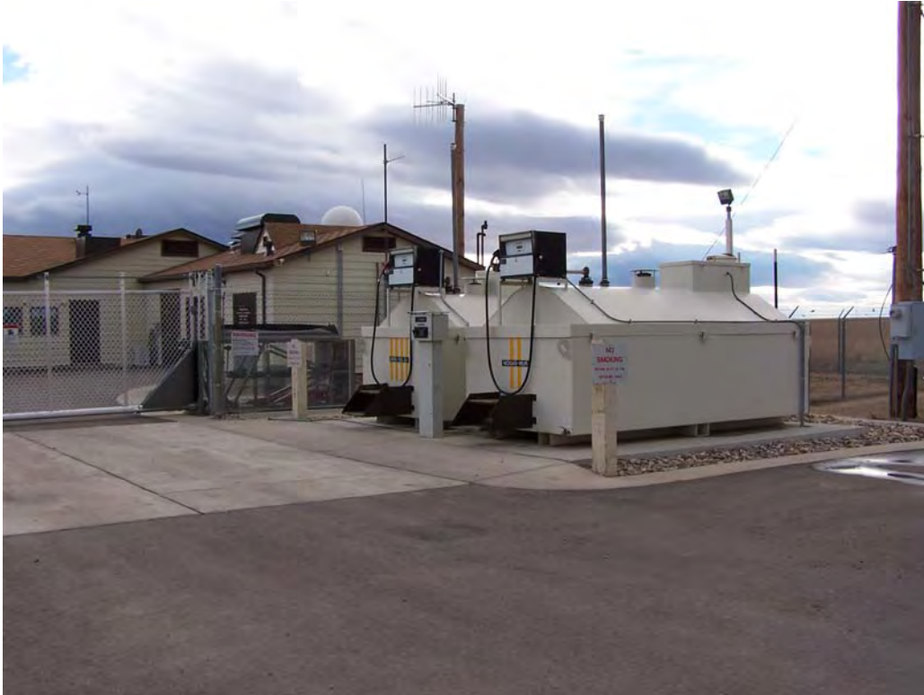
Photograph A-7. MAF J-1 ASTs outside fenceline.
